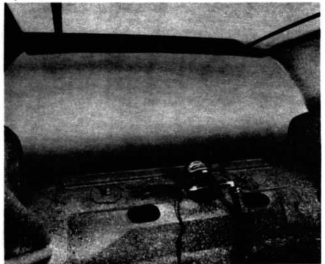
FIGURE 28. Welded-In Plate Between Trunk and Rear Seat Area.
